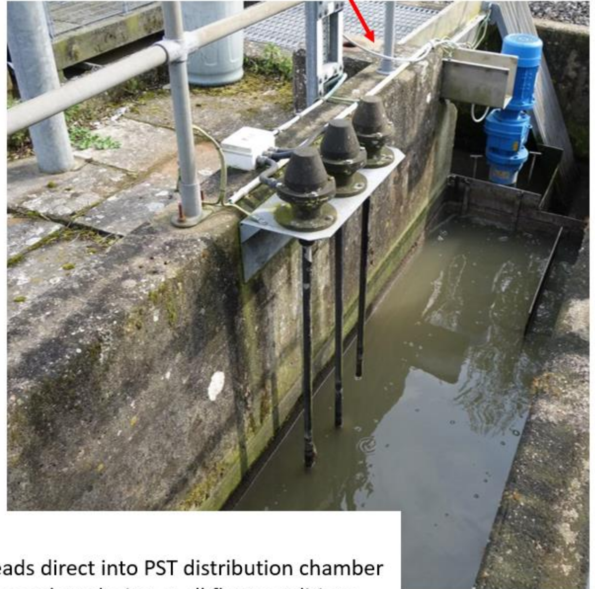
PST distribution chamber
